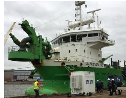
Harbor Power Supply
